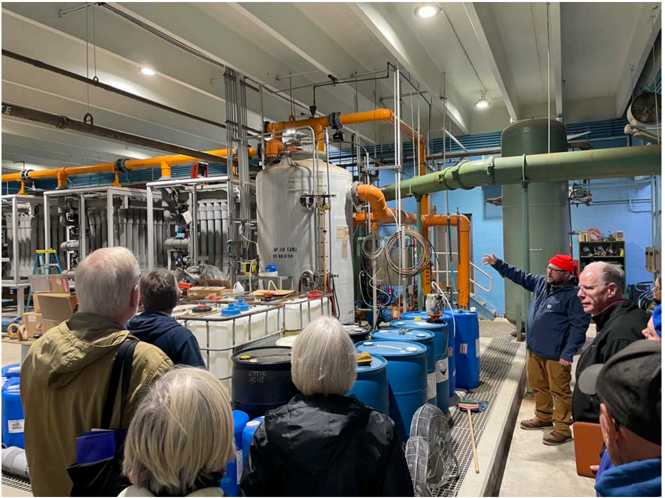
2 Summit attendees had the unique opportunity to tour the water treatment plant on Mackinac Island
